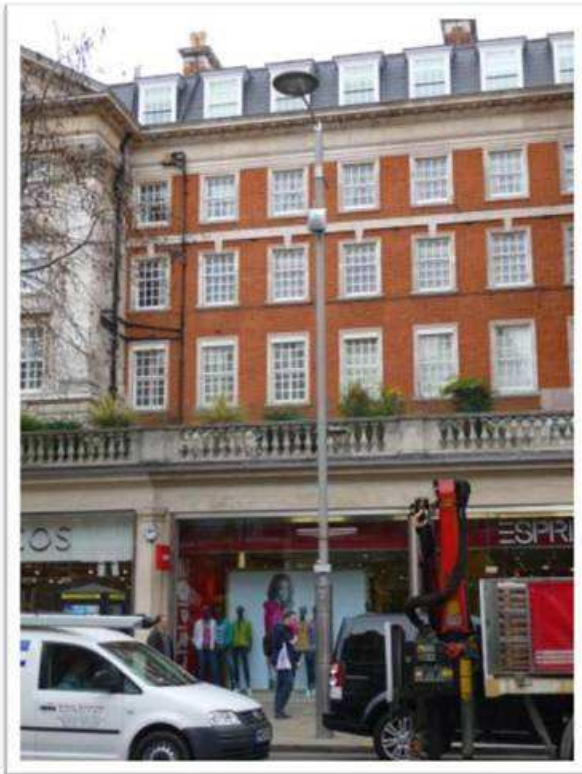
Figure 1 - Rukus 8800 installed in Kensington High Street
